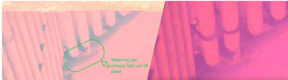
1. Retaining bar out of place
