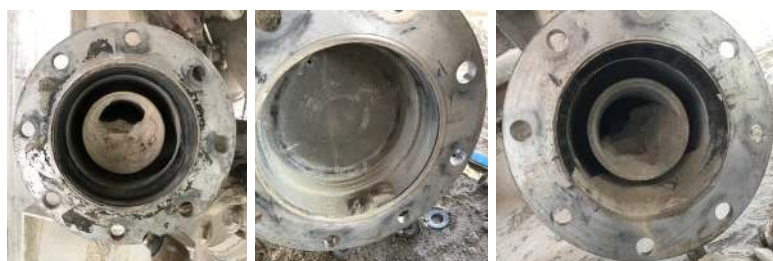
Figure 3. Original damaged parts: clinker filled air cannons.
