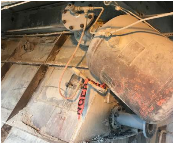
Figure 4. IGS Retrofit 6 months in operation.
