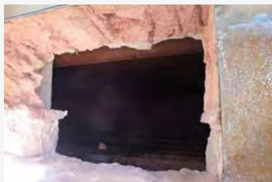
Figure 3. The external casing was cut up and a rectangular opening was created.
