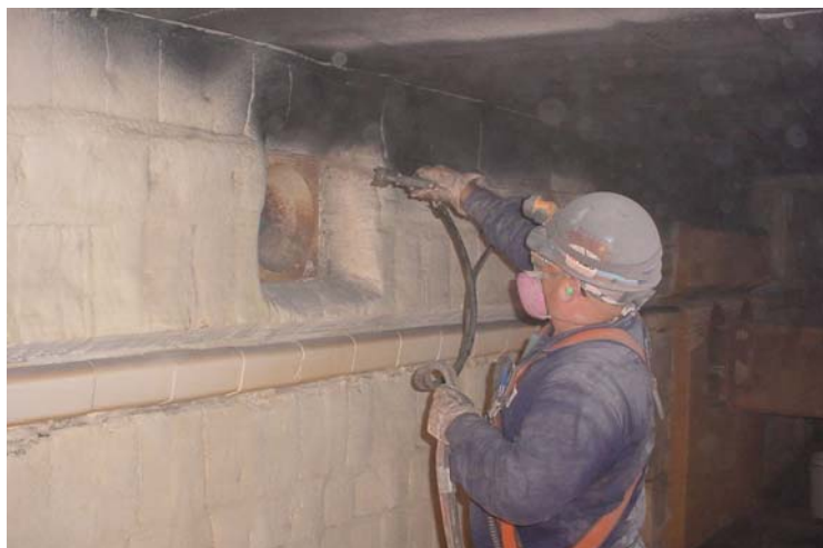
Figure 6. High Emissivity Coatings Applied to Ceramic Refractory Fiber
