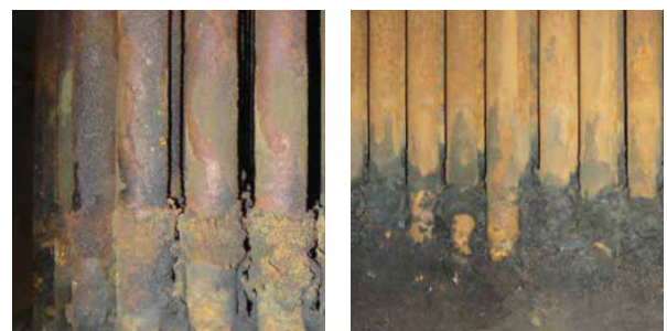
Shell Side Fouling Showing Corrosion and Hard Coke Deposits
